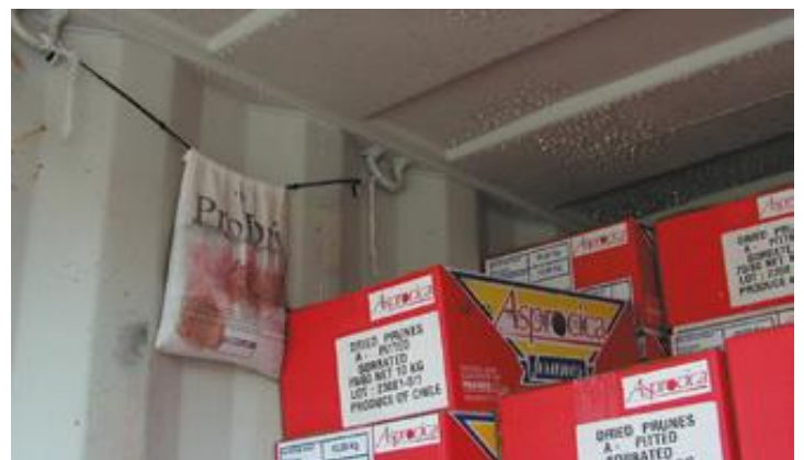
Condensation water on roof, dry bag already completely soaked
